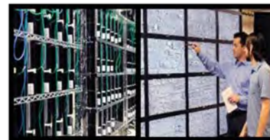
High Performance Computing Facility
