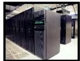
Corporate Research and Development Server Facility (CRDSF)
